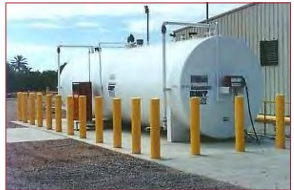
1 - Above Ground Storage Tank
