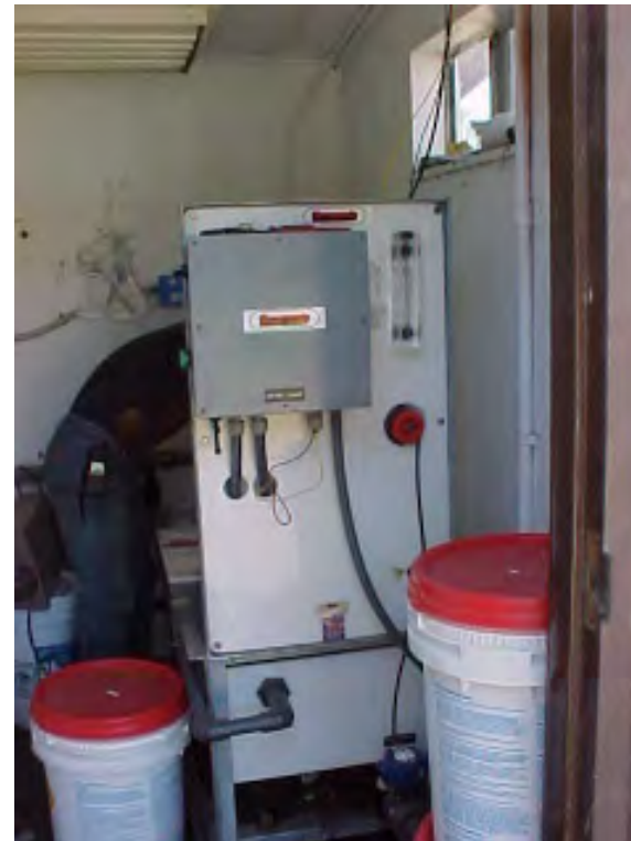
A Chlorination System
