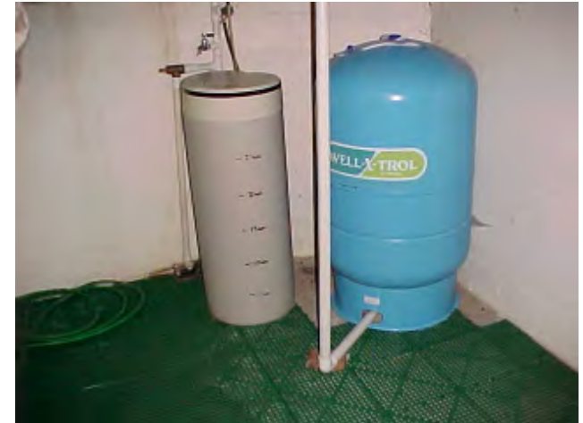
A Hydropneumatic Storage Tank
