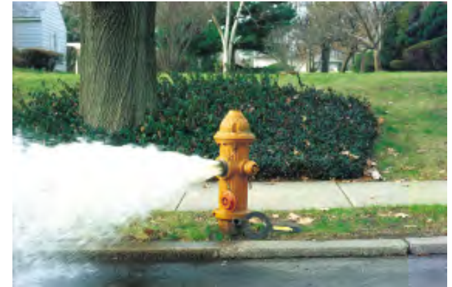
Hydrants Provide Water for Fire Suppression, Line Flushing, and Irrigation
