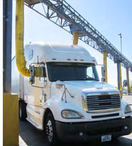
A typical overhead gantry-based TSE system providing HVAC, electrical, and internet services to a long-haul truck.
