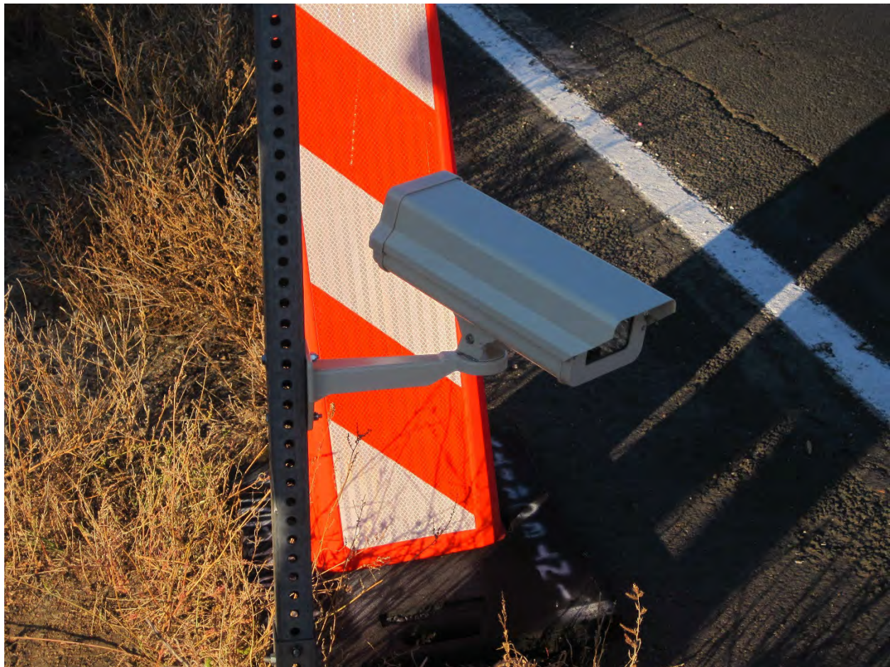
Figure 2-5. Video Camera Installed Near EDAR System
